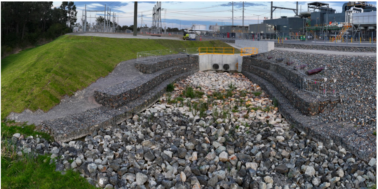
Figure 8.2: KKPS stormwater discharge outlet
