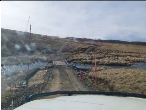
GTS15: Tantangara Creek crossing – high flowing water
