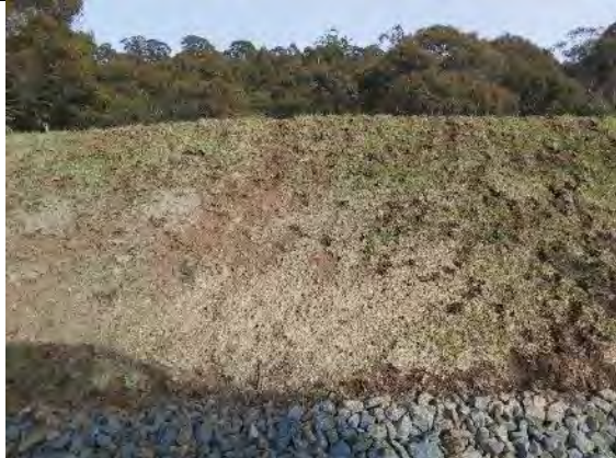
TT11: Hydromulched stabilised batter – damage by brumbies
