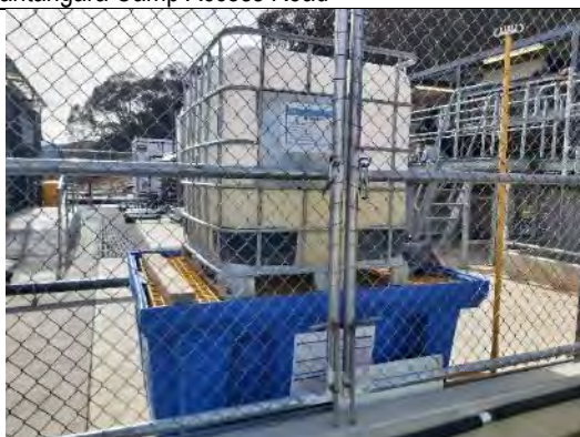
TT15: Sewage Treatment Plant (STP)– Tantangara Camp
