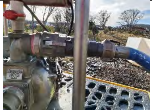
MC25: Leaking hose fitting
