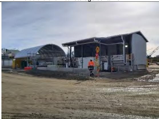
TT28: Fuel Farm at Fill 2
