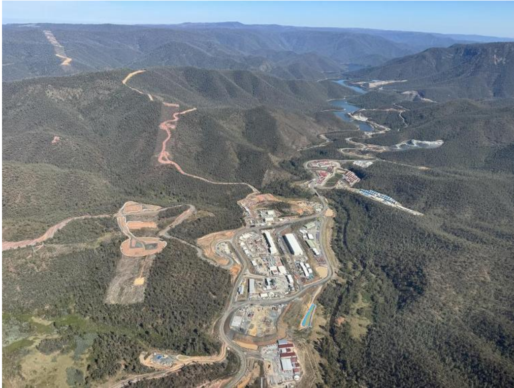
Figure 7.8: Lobs Hole works area that forms part of the Snowy 2.0 project within Kosciuszko National Park, NSW. Photo by Z. Atkins.
