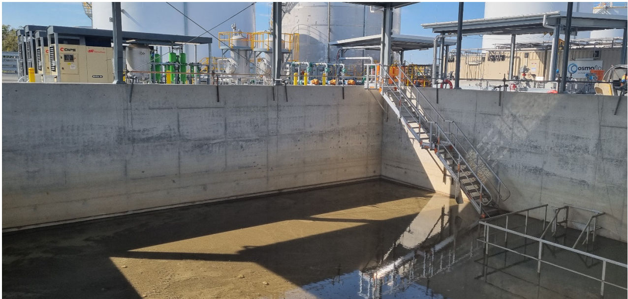
Photograph 7: Permanent oil pit interceptor utilised for site runoff
