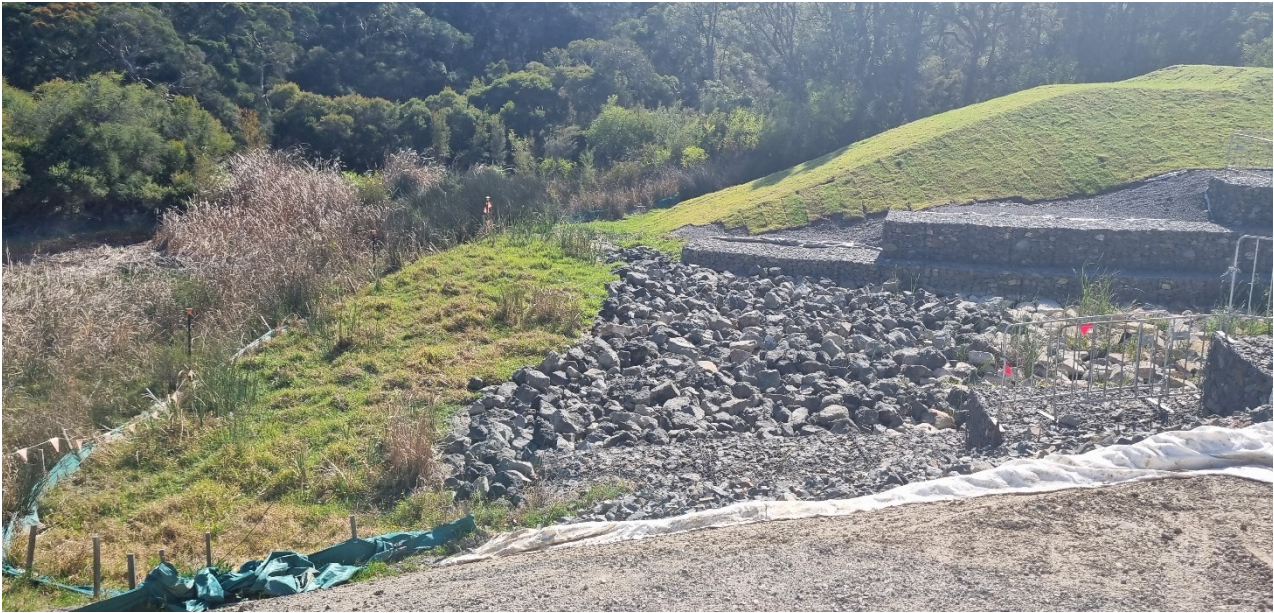
Photograph 9: Surface water discharge structure
