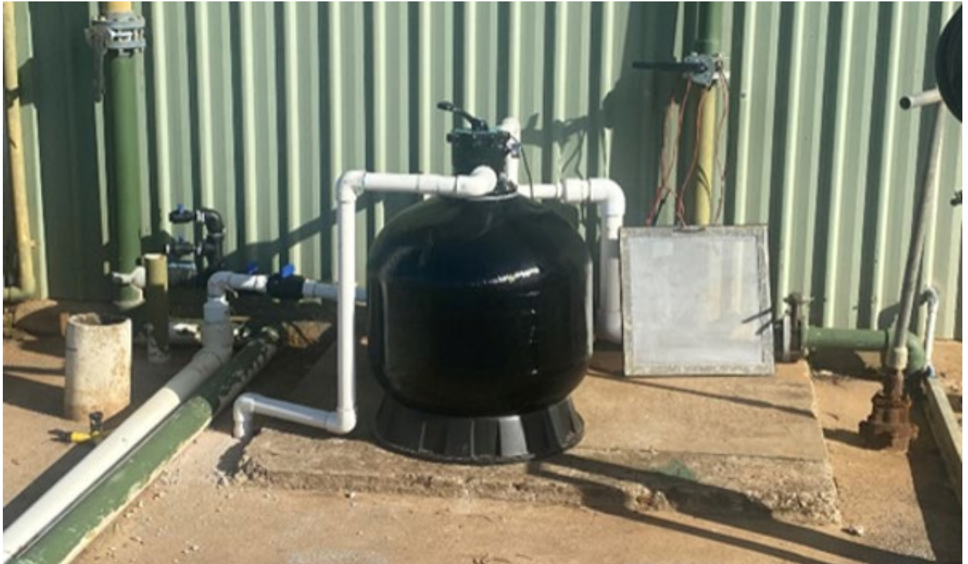
Figure 17. New sand filter installed on river line.
