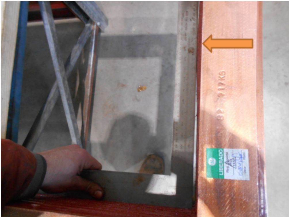
Previous dimensional non-conformance on a new winding that prevented the winding fitting onto the pole body
