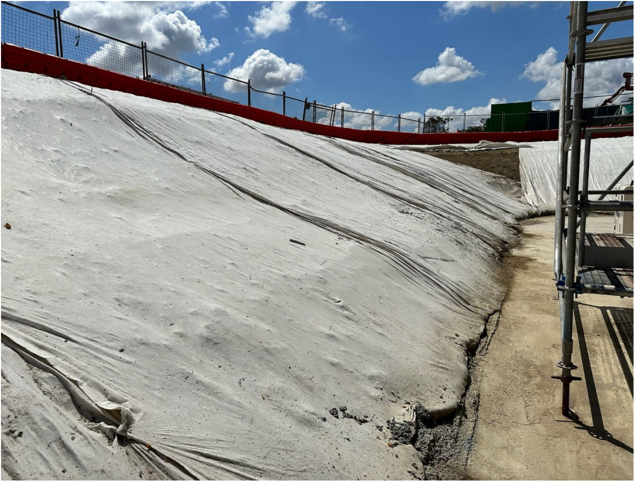
Photograph 5 – Geofabric erosion protection, oil water separator embankment
