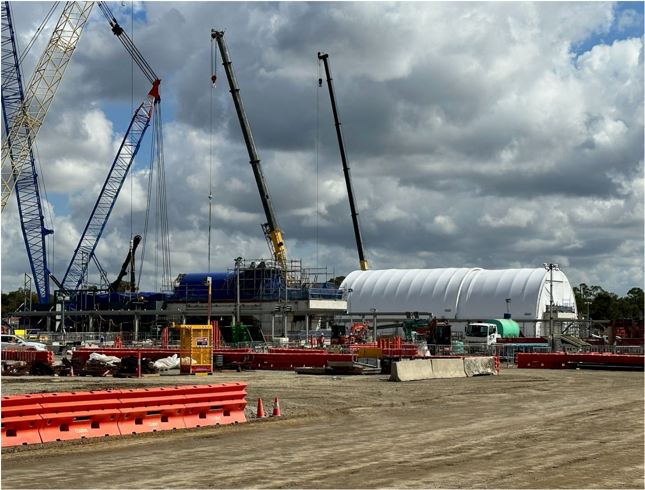
Photograph 3 – Construction of turbine base and controlled clean room environment for installation of mechanical components
