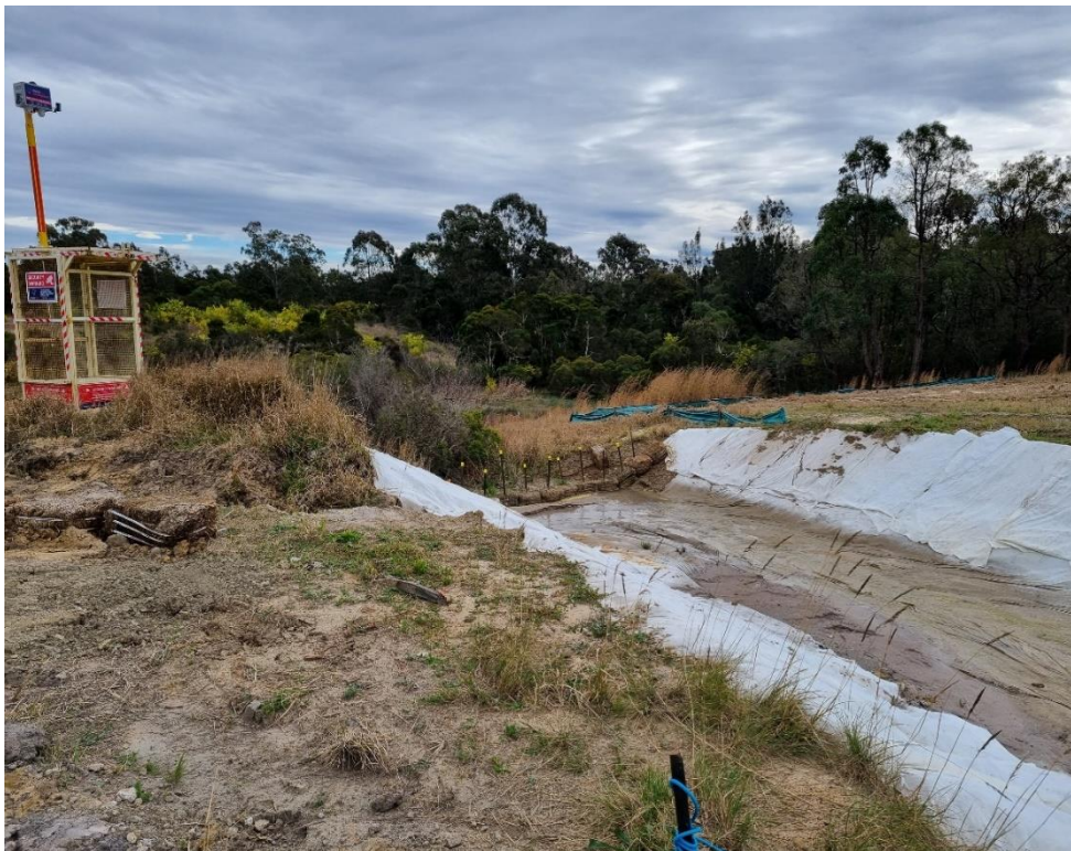
Photograph 5 - Lined discharge channel from sediment pond (and WWTP)
