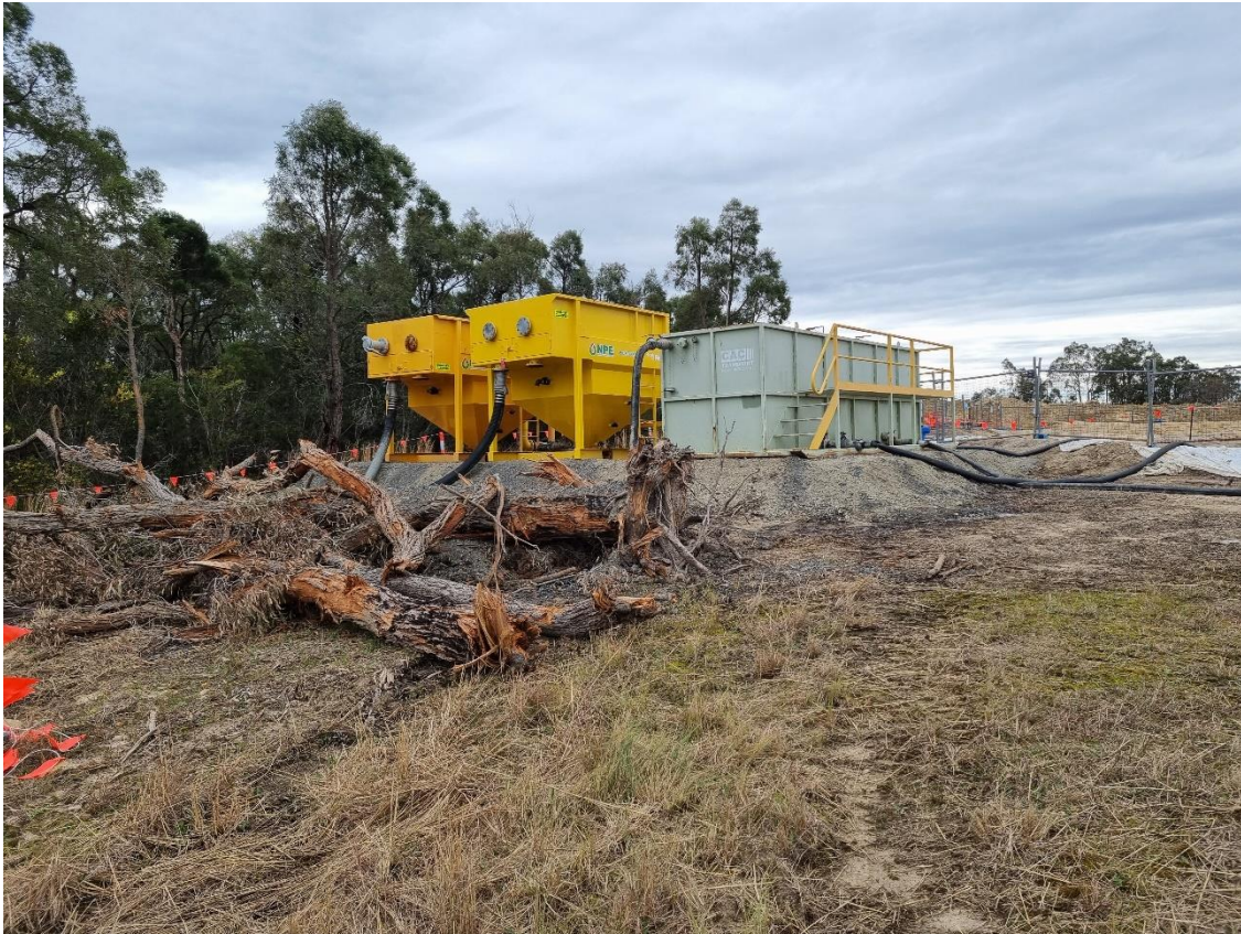
Photograph 7 - Wastewater Treatment Plant
